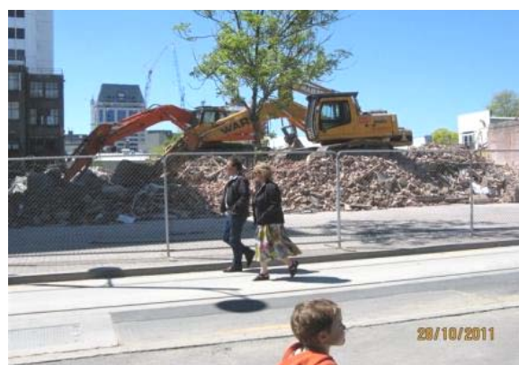
Above: What remains of "the strip"; the area on Oxford Terrace that was similar to the Hood Street bar/café area
